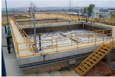
Sequencing Batch Reactor (SBR)
