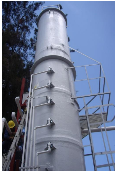
EGSB Aerobic reactor
