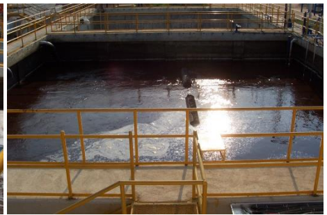
Sequencing Batch Reactor (SBR)
