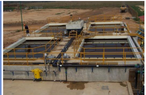
UASB Anaerobic reactors
