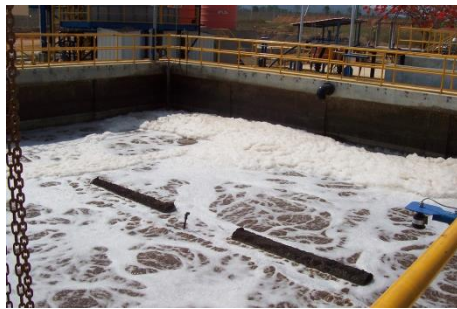
Sequencing Batch Reactor (SBR)
