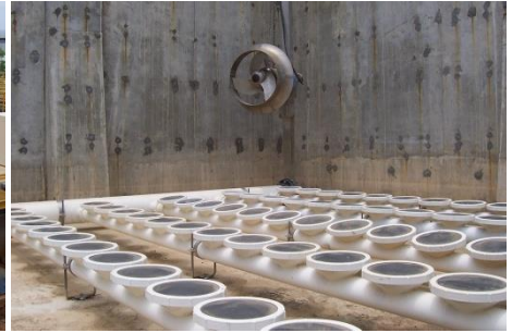
Interior of aerobic reactor
