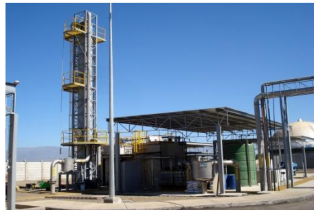
System for washing biogas
