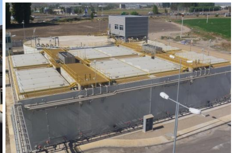
UASB anaerobic reactors
