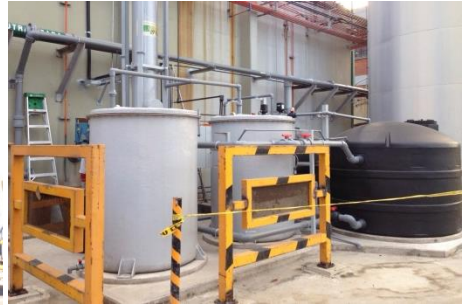
Scrubber and compost biofilter for odor control
