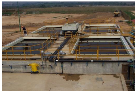
UASB anaerobic reactors
