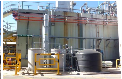
Scrubber and compost biofilter for odor control
