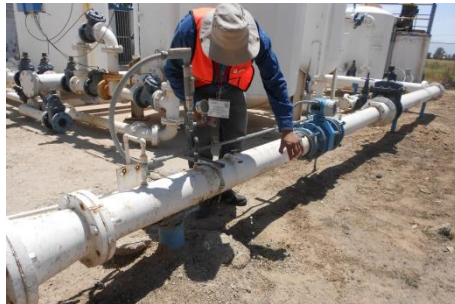
Evaluation of the physical conditions of 234 WWTPs with capacity less than 100L/s
