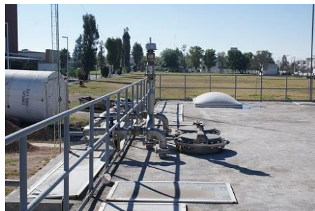
Output of biogás from UASB anaerobic reactors
