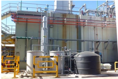
Scrubber and compost biofilter for odor control
