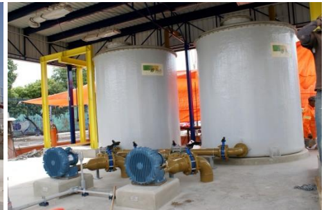
Compost biofilter for odor control
