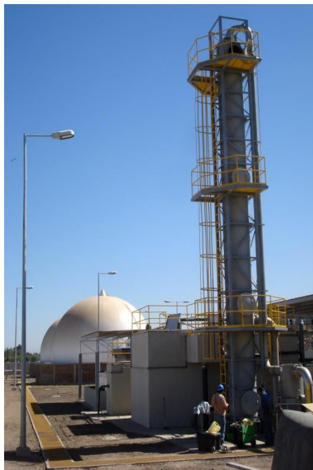
Biogas washer system
