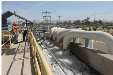
Evaluation of the physical conditions of 234 WWTPs with capacity less than 100L/s
