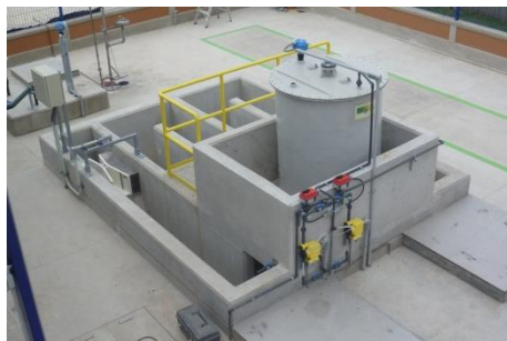
Contact tank with chlorine
