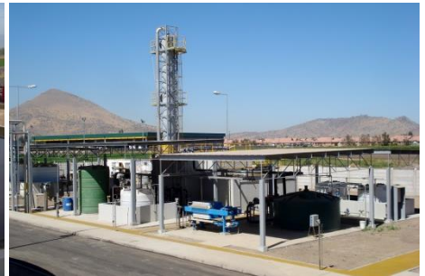
Biogas washer system
